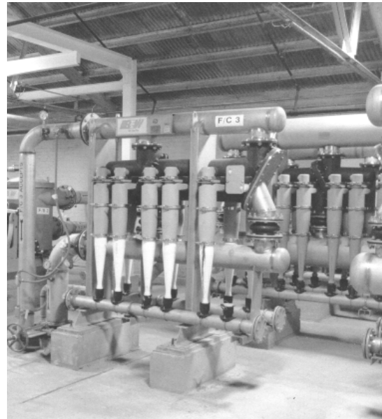
Banks of centrifugal cleaners remove high specific gravity contaminants.
